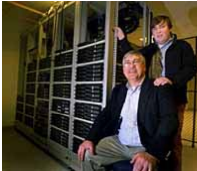
Wayne Sawchuk and his son, Aaron Sawchuk, founded ColoSpace, a company that provides data backup and disaster recovery for clients. ColoSpace is opening its fifth data center in Rockland next month. (GREG DERR/The Patriot Ledger)
